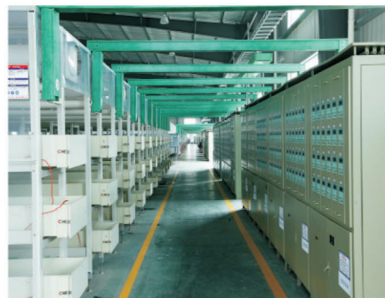
内化成充电系统 Internalized Charging System
